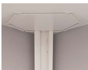
Fire seals for both levels
